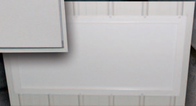
Installed Door View
